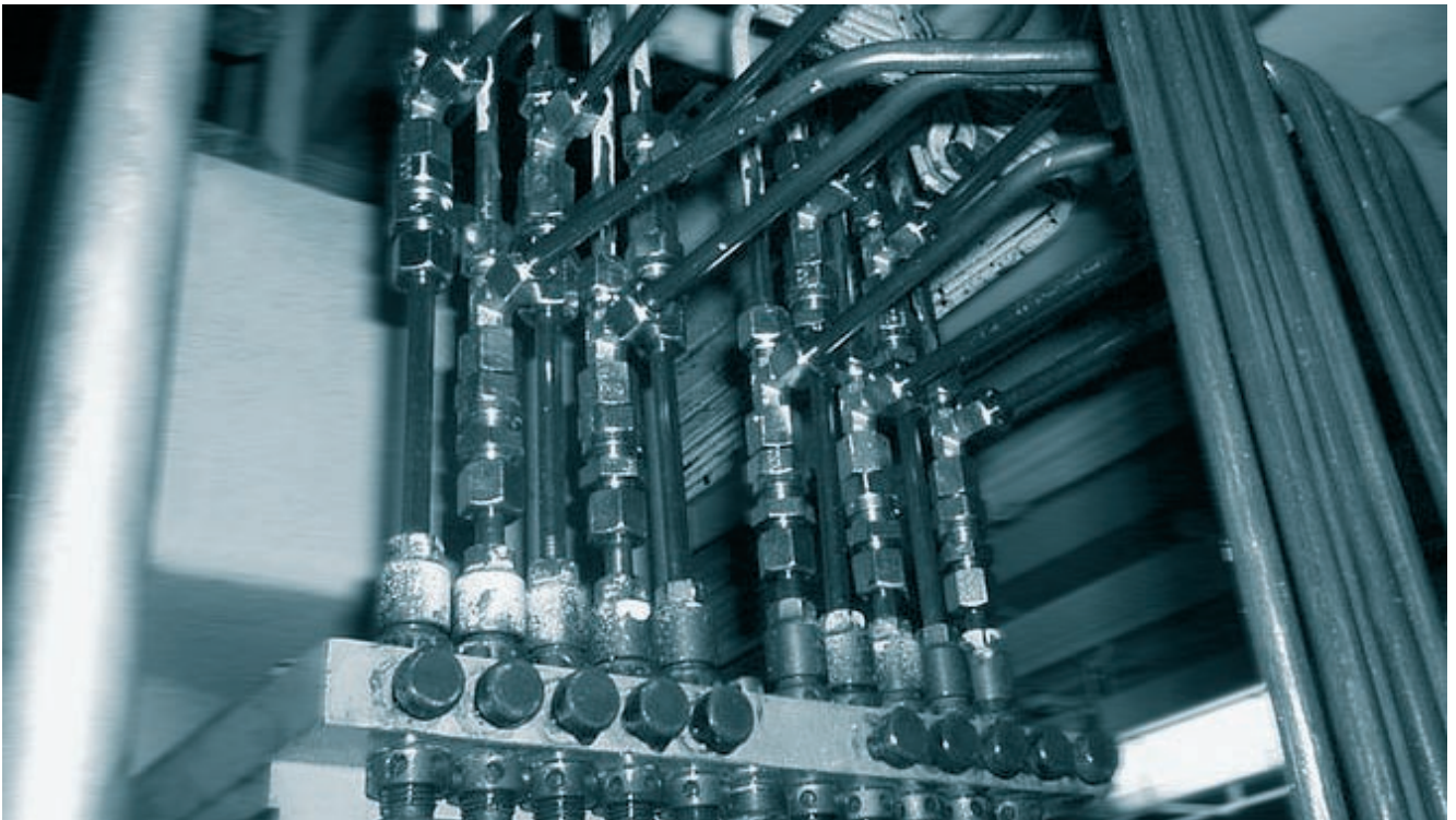
Insertion of non-return valves and T- piece (position 4) with end plug in existing lubricator piping
